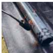
Expansion joints performing
